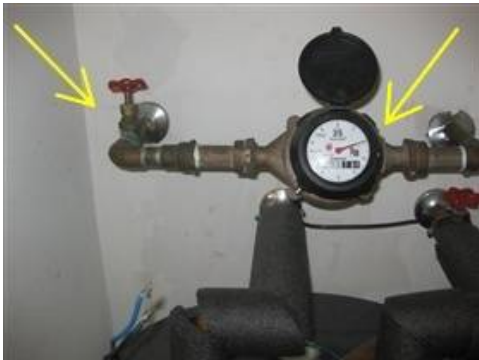
Photo X-3 Main water shut off and water meter
