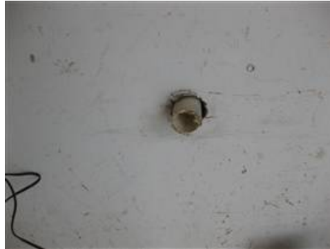
Photo X-2 uncapped pvc pipe in garage
