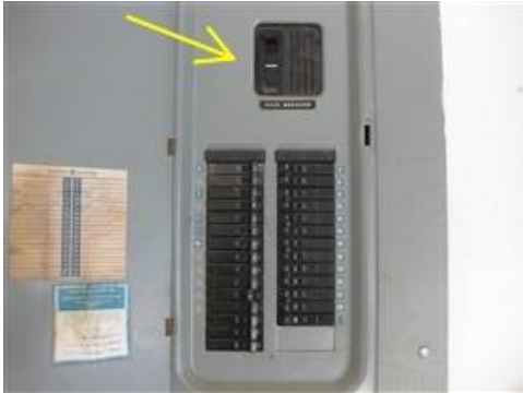
Photo X-1 Main electric shut off
