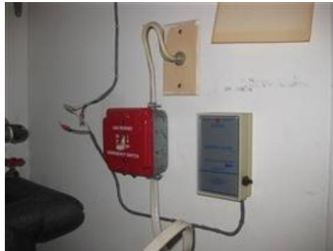
Photo X-4 Electric water heater shut off
