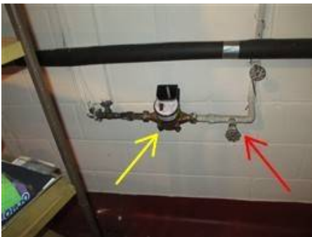
Photo X-5 Water meter & Main water shutoff
