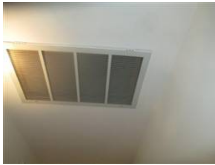
Photo X-10 2nd floor A/C filter behind grill
