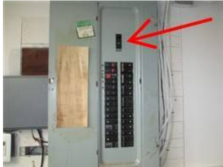
Photo X-4 Main electric shutoff
