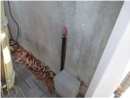
Photo X-1 Unknown wire protruding from ground near electric meter
