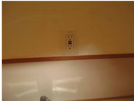
Photo 23-2 Bar sink area
