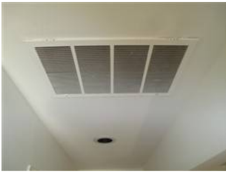
Photo X-9 1st floor A/C filter behind grill
