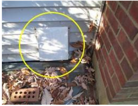
Photo X-2 Exhaust vent for kitchen range
