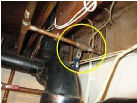
Photo X-7 Shutoff for rear hose bib
