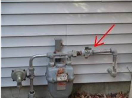
Photo X-3 Main gas shutoff
