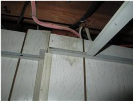
Photo 43-3 Above Main electric panel
