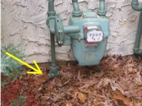
Photo X-1 Main Gas shut off
