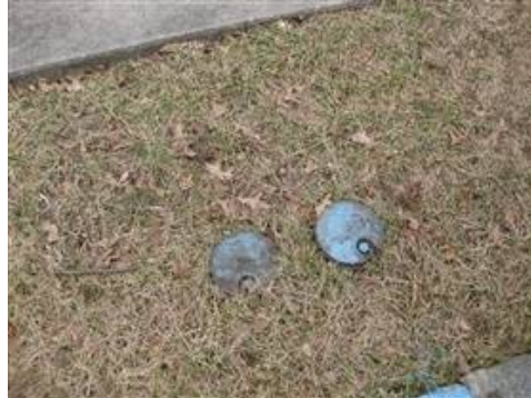
Photo X-2 Main water shut off on street
