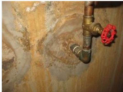
Photo X-4 Main water shut off in Basement
