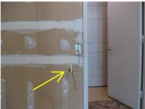
Photo X-5 Reset for all bathroom GFCI outlets
