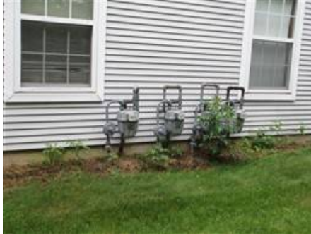
Photo X-2 Main Gas Shut-off
