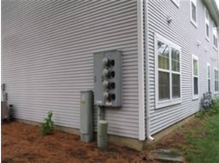
Photo X-1 Main Electric Shut-off
